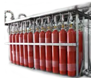
CO2 Extinguishing System
